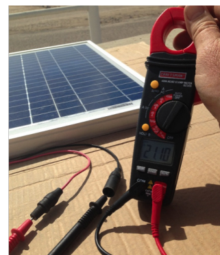
Figure 2. The open-circuit voltage (Voc) of a 20-watt solar PV module is measured connecting the positive lead of the meter to the positive connector, and the negative lead to the negative connector. The reading is 21.10 Voc in full sun during the middle of the day. In this photo, a digital clamp-on ammeter with leads is used to perform the circuit measurements. Source: Author
