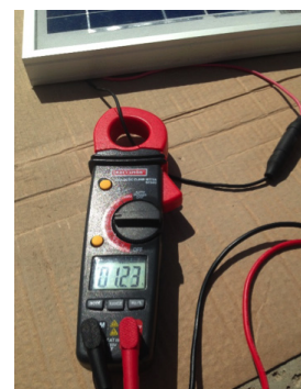
Figure 6. Measuring the short-circuit current (Isc) of a 20-watt solar module with a digital clamp-on meter. The module leads are connected together and the meter clamp encircles one of the conductor leads. The reading is DC current of the module when there is no load. Source: Author
